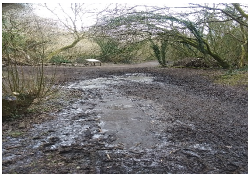
Full length of the path to be scraped and stone added to address the drainage issues
